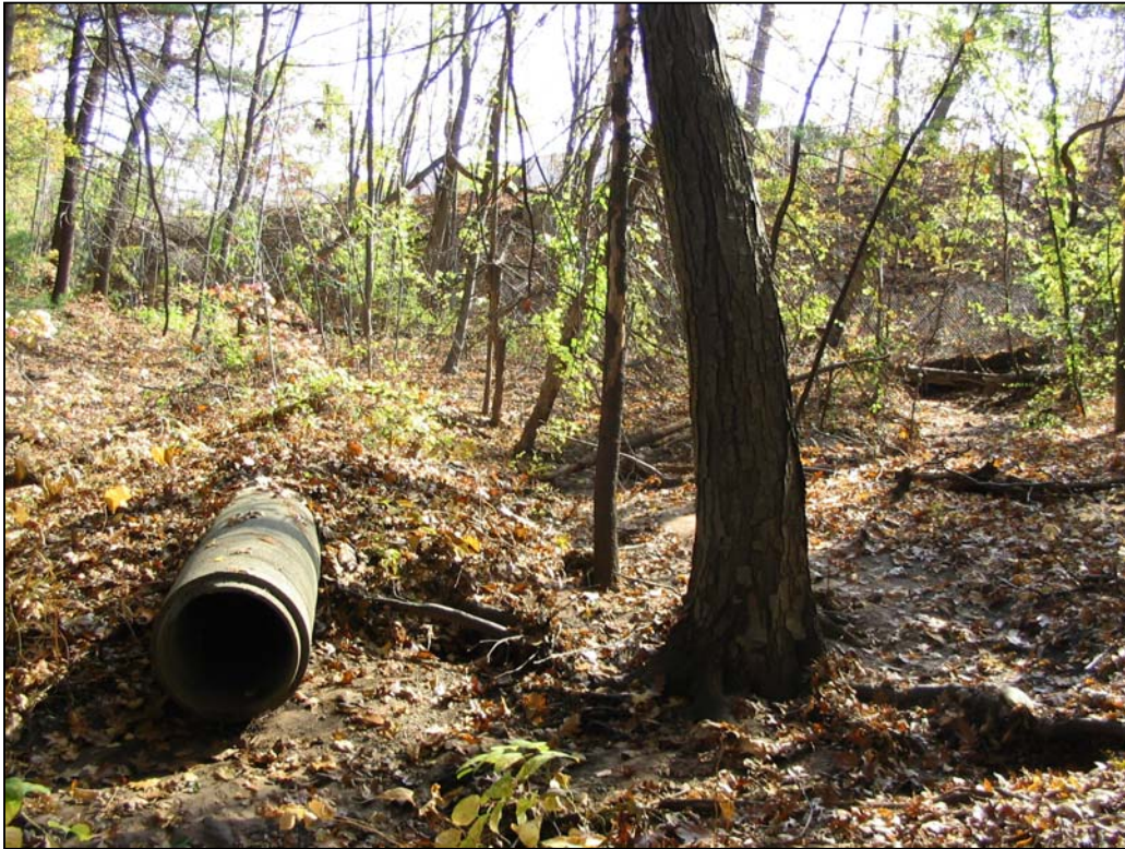
Current stormwater drainage systems on site are in disrepair, causing severe erosion, as shown in this photo of urban runoff entering Pond C via a stream rather than the intended aqueduct.
