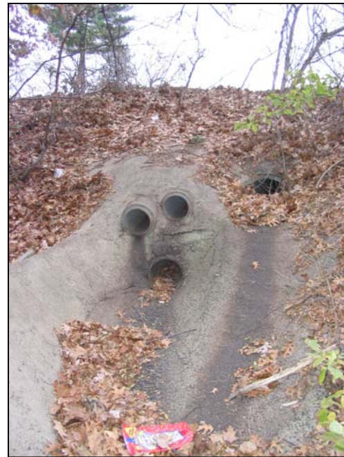
Stormwater outflow pipe that drains onto the Olin Powder Farm property.
